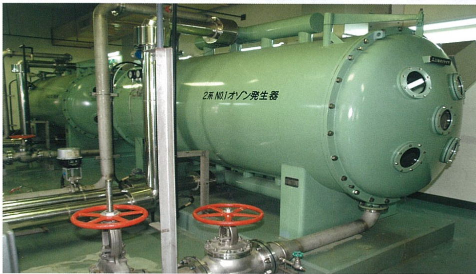
Advanced Water Treatment Facilities
