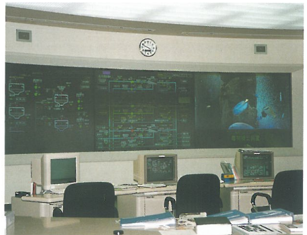
Central Control Room
