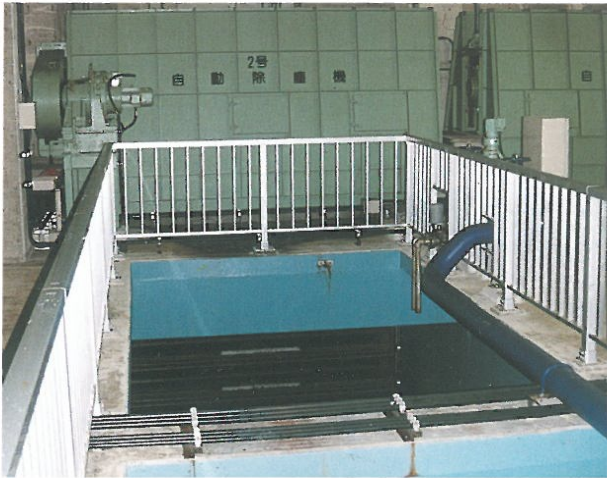
Sand Settling Basin
