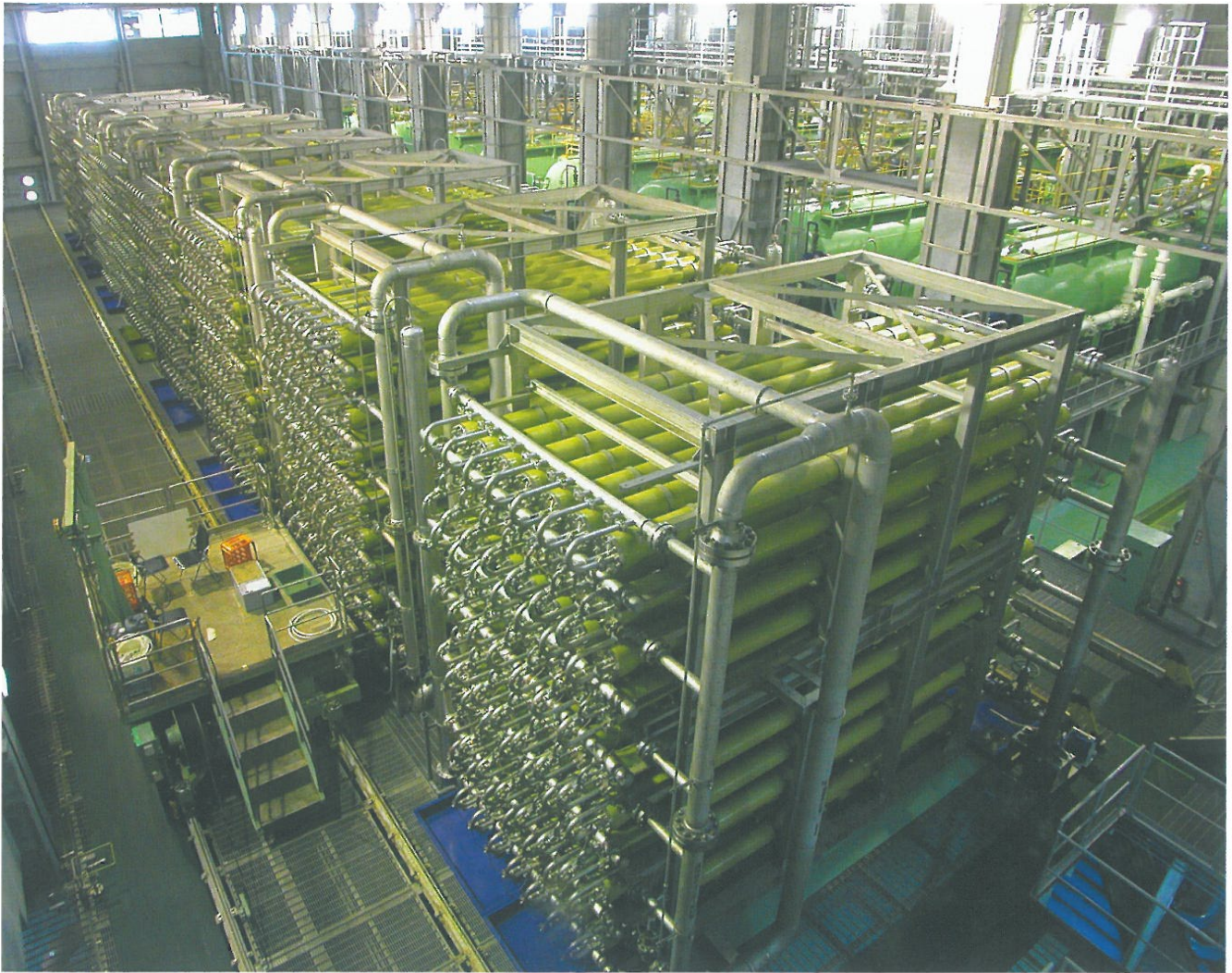
Reverse Osmosis Membrane Units
