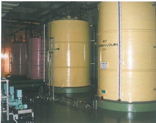
Chemical Feeding Room
